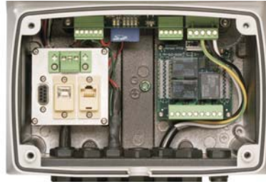
FRONT COVER PLATE REMOVED
